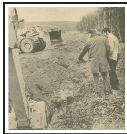
Sewage system concerns halted construction
